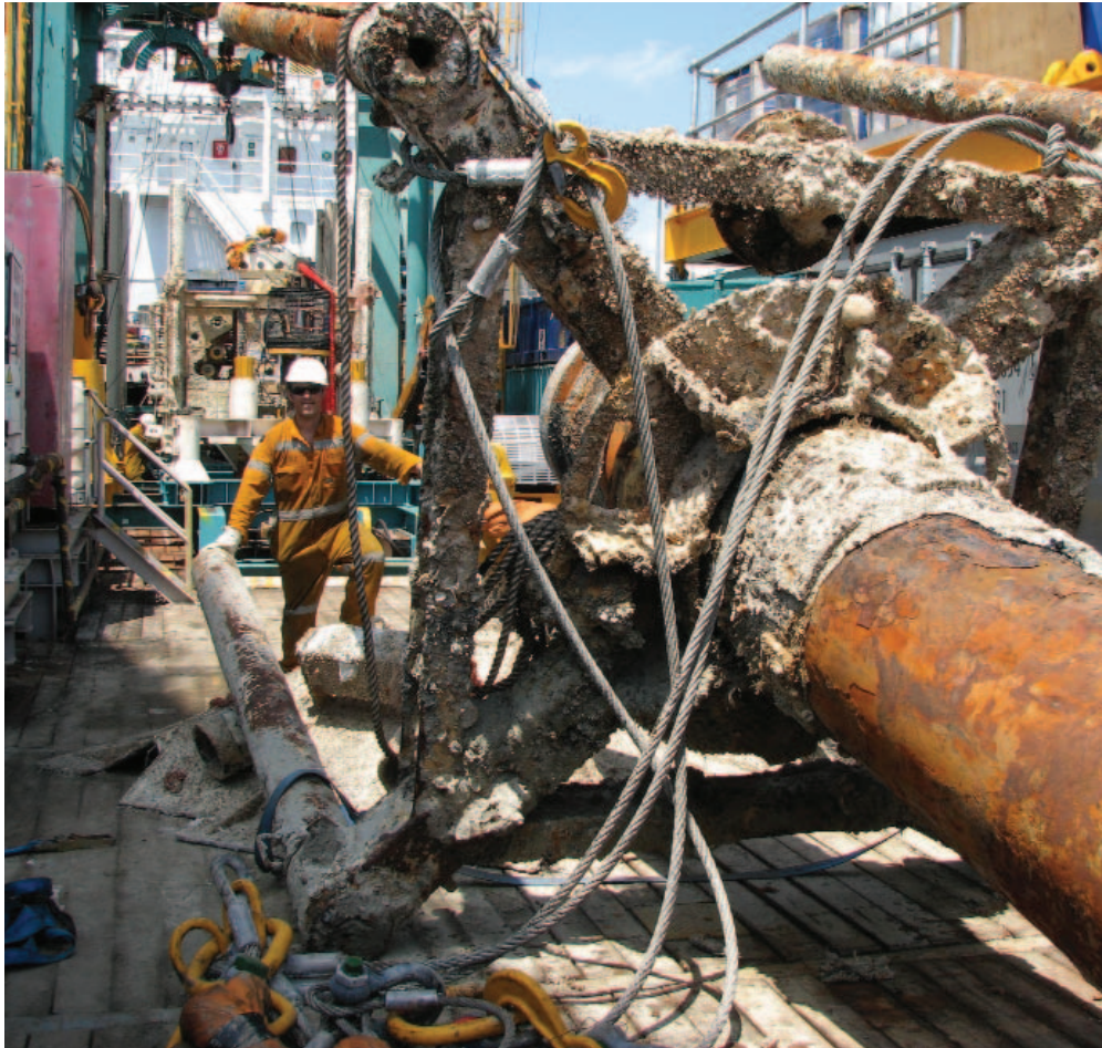
Figure 2. The wellhead was removed successfully in what possibly could be the world's deepest rigless subsea well abandonment.
